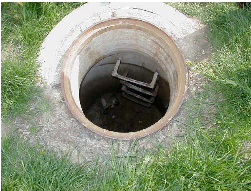
Figure 1. The landfill manhole where the fatality occurred.
