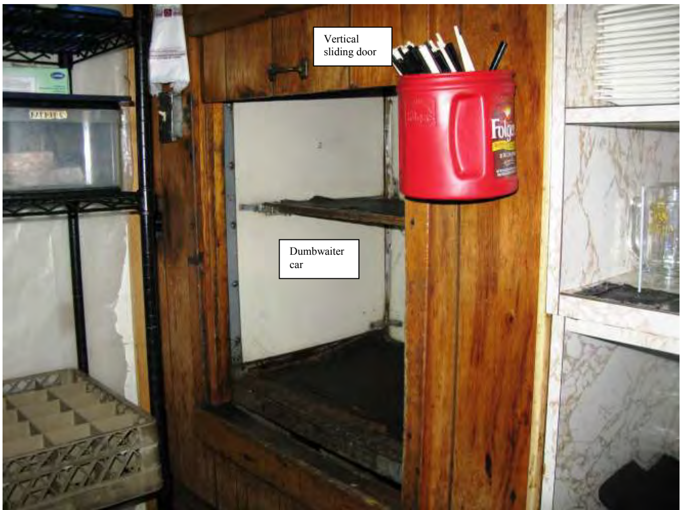
Photo 1. The hoistway door opening in the upstairs food preparation area with the dumbwaiter car in the landing zone. The sliding door was nailed to stay in the up and open position.
